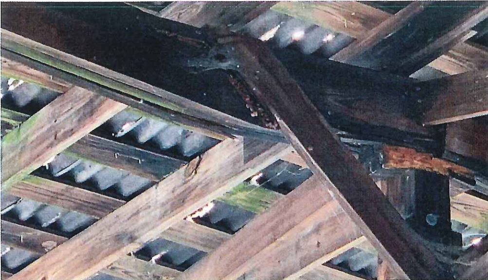
Image: A roofing support beam on L-dock has completely failed due to rot. The damaged beam was replaced at a cost of $9,000.
